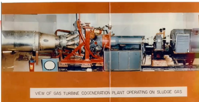
VIEW OF GAS TURBINE PLANT OPERATING ON SLUDGE GAS
